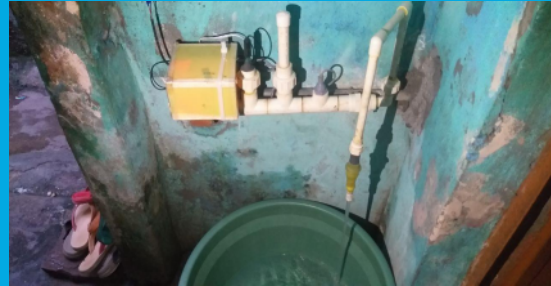
Water Quality monitoring sensor assembly installed at Location-2
