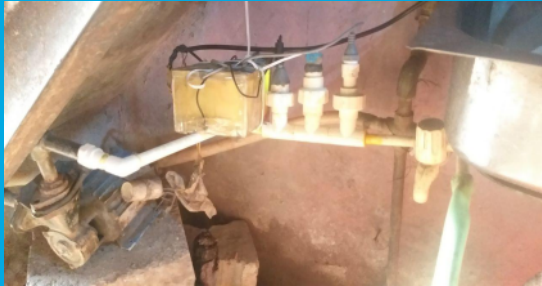
Water Quality monitoring sensor assembly installed at Location-1
